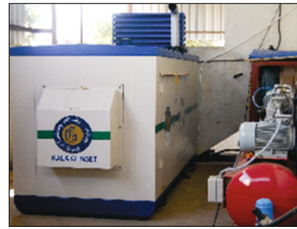
Captive Power Arrangement Diesel Silent Generator (Kala Genset) - 82.5 KVA
