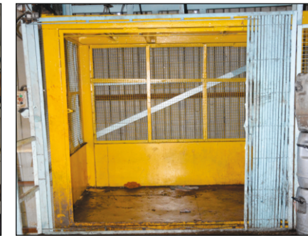
Material Lift Facilities
